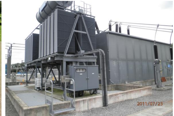
400 kV Power Transformer
